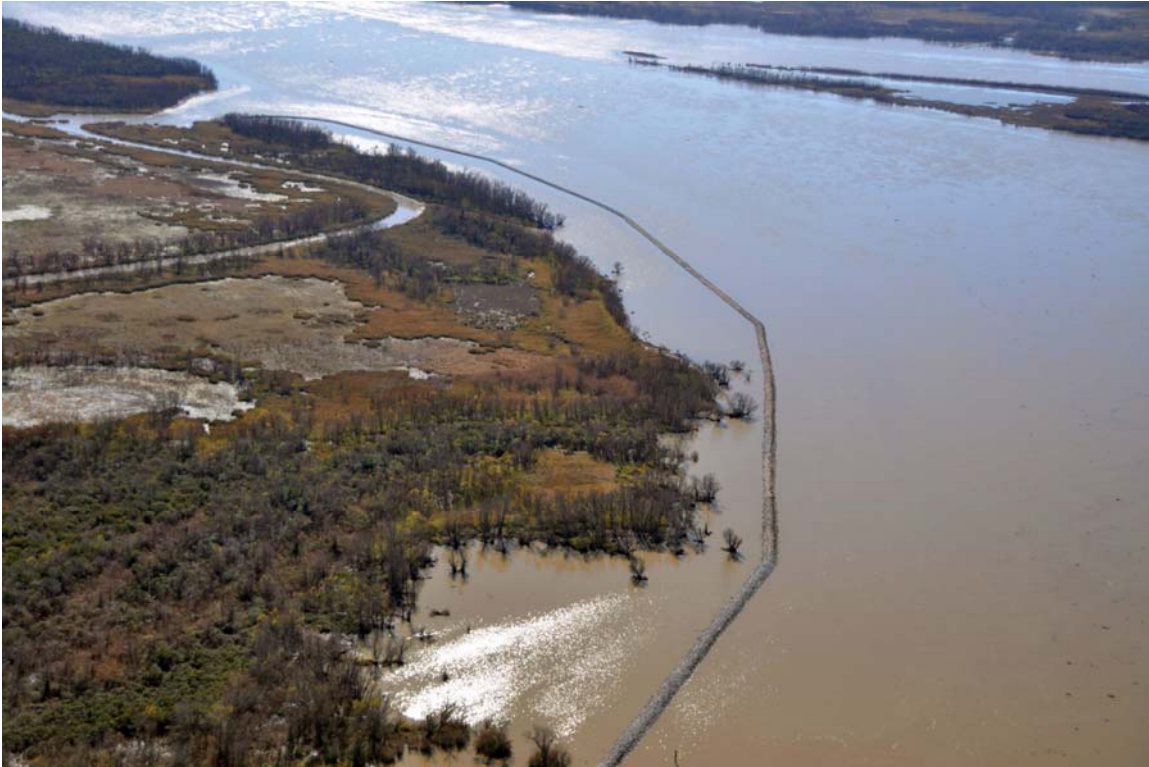
Figure 2-2: Crew Boat Cut Revetment as seen from the air, looking towards the southwest (photo credit: Greg Linscombe)
