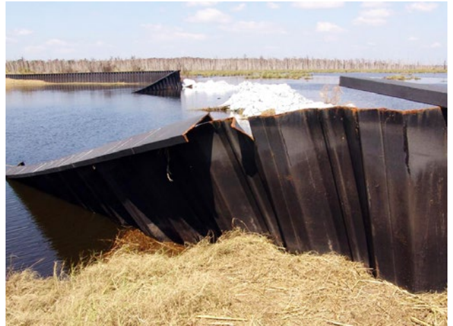
Levee Breach Wonder Lake levee breach resulting from Hurricane Rita. Photo Credit: FEMA/Greg Henshall
