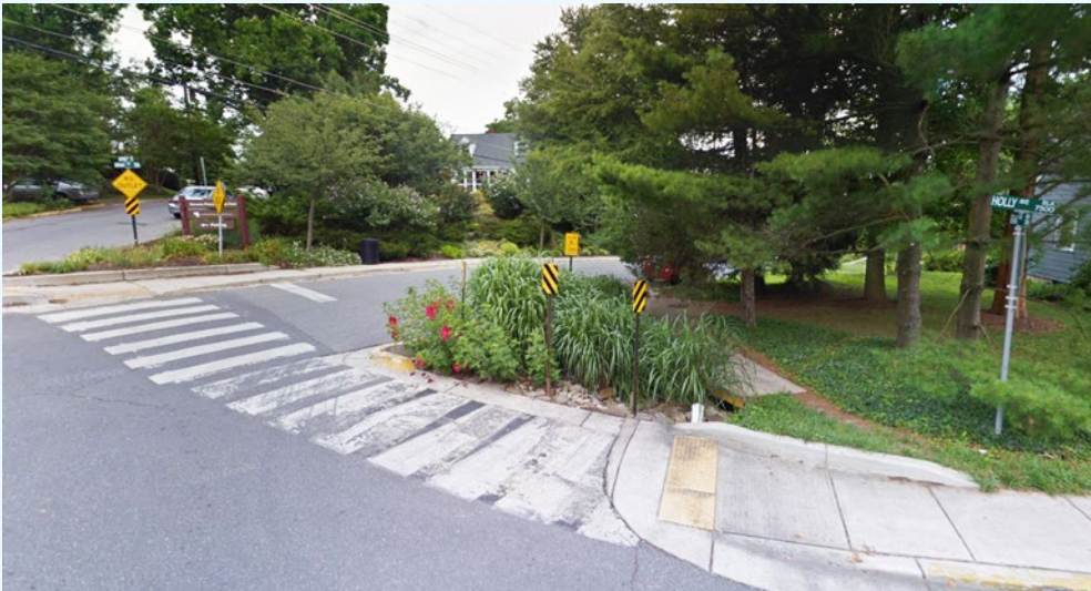
Grant Ave. bioretention cells, curb cuts, and ADA-compliant sidewalk upgrades. Photo Credit: Google Maps Street View
